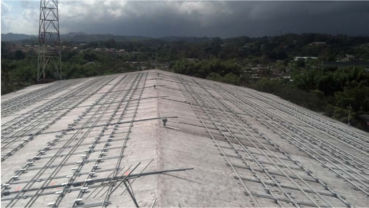
Figure 1. Commercial Scale Enphase Project
